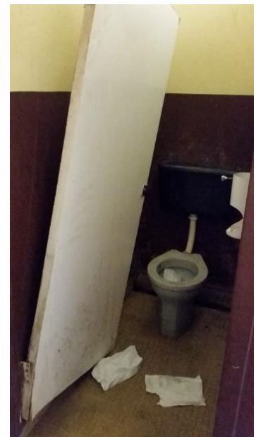
Figure 1. Toilet in a primary school in Port Elizabeth, South Africa. October 13, 2017.
